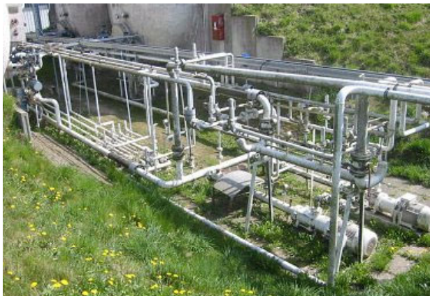
Figure 5. Pipelines of company Boie in Lübeck
